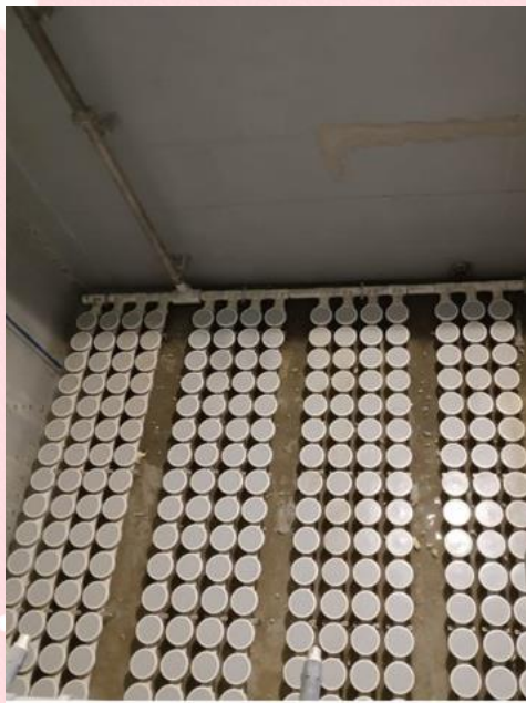
Installation of air diffusers in Sludge Digestion Tank 污泥消化缸內好氧處理系統安裝工程
